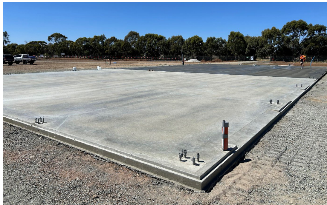
Freshly poured concrete slab at the Automated Depot shed Moama Waste Management Facility
