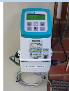
New filtered flow meter at Mathoura WTP
