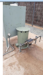
Odour control unit at pump station
