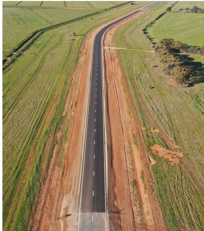
Drone imagery of completed Wakool Road reconstruction (Ch: 27km). Great finish to the works despite some uncontrollable delays with ground conditions and weather.
