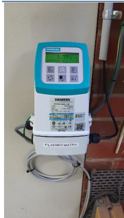
New filtered flow meter at Mathoura WTP
