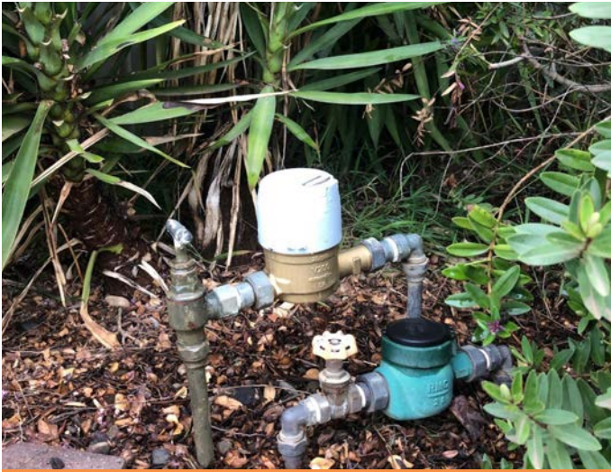
Smart meters were installed at over 6500 properties
