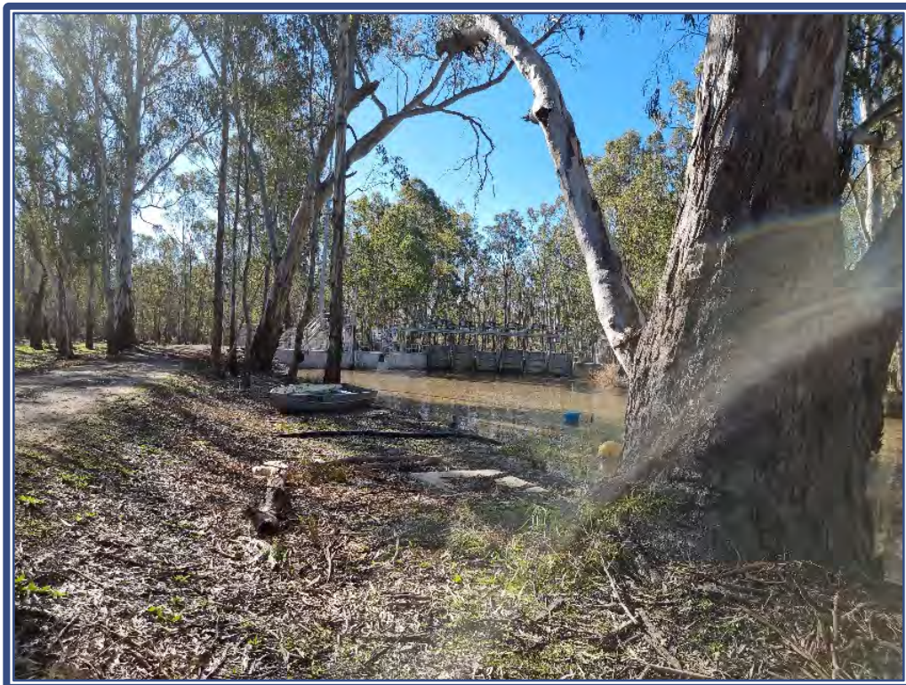
Figure 2-4 Pump suction pipe through levee bank looking downstream
