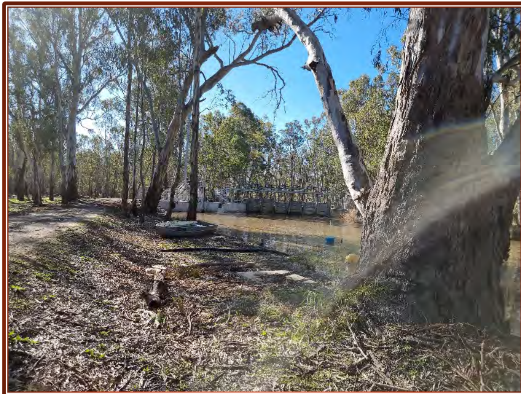
Figure 3-4 Pump suction pipe through levee bank looking downstream
