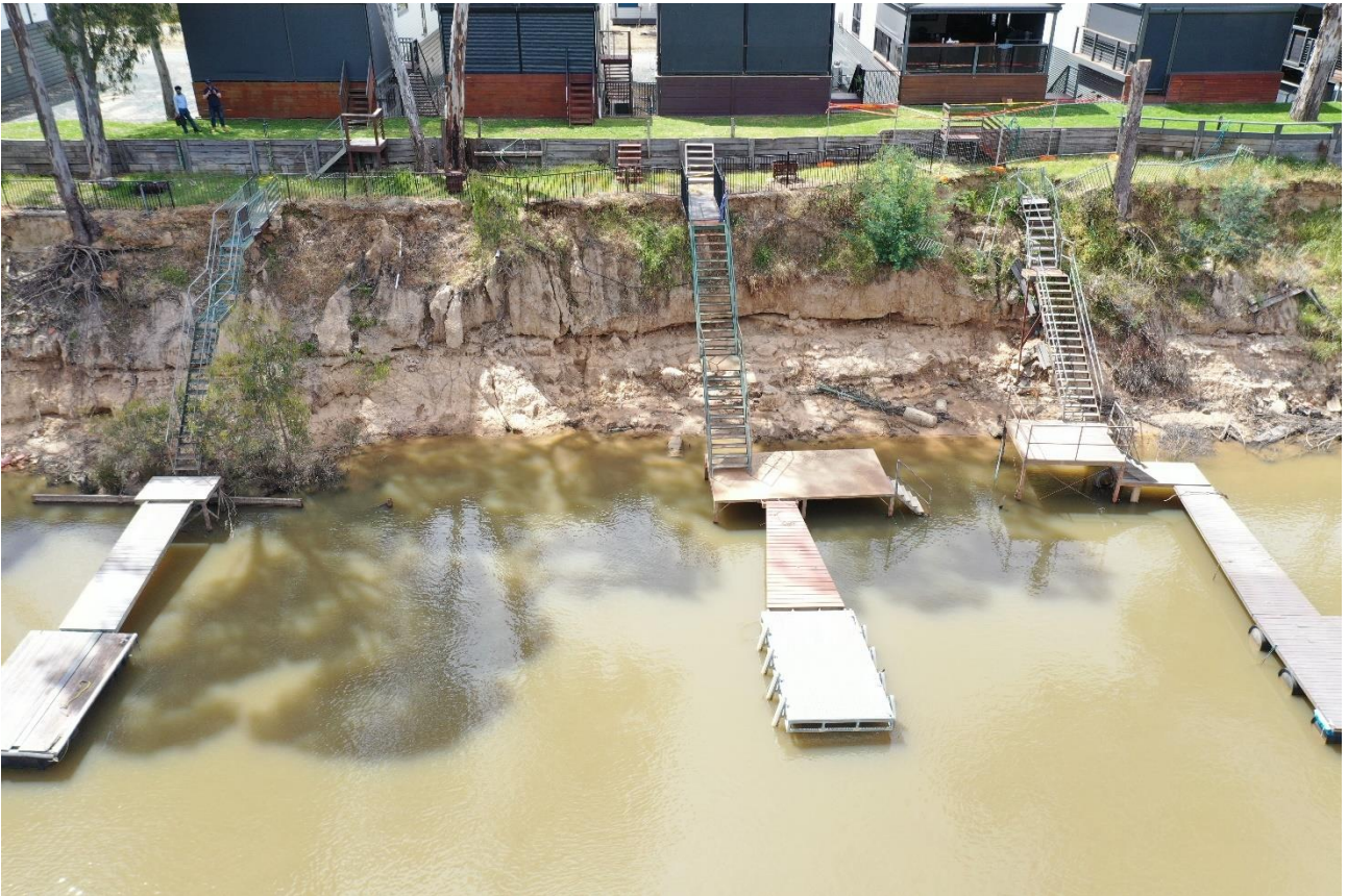
Figure 3: Site 2 – riverbank erosion (undercutting, leading to mass failure)
