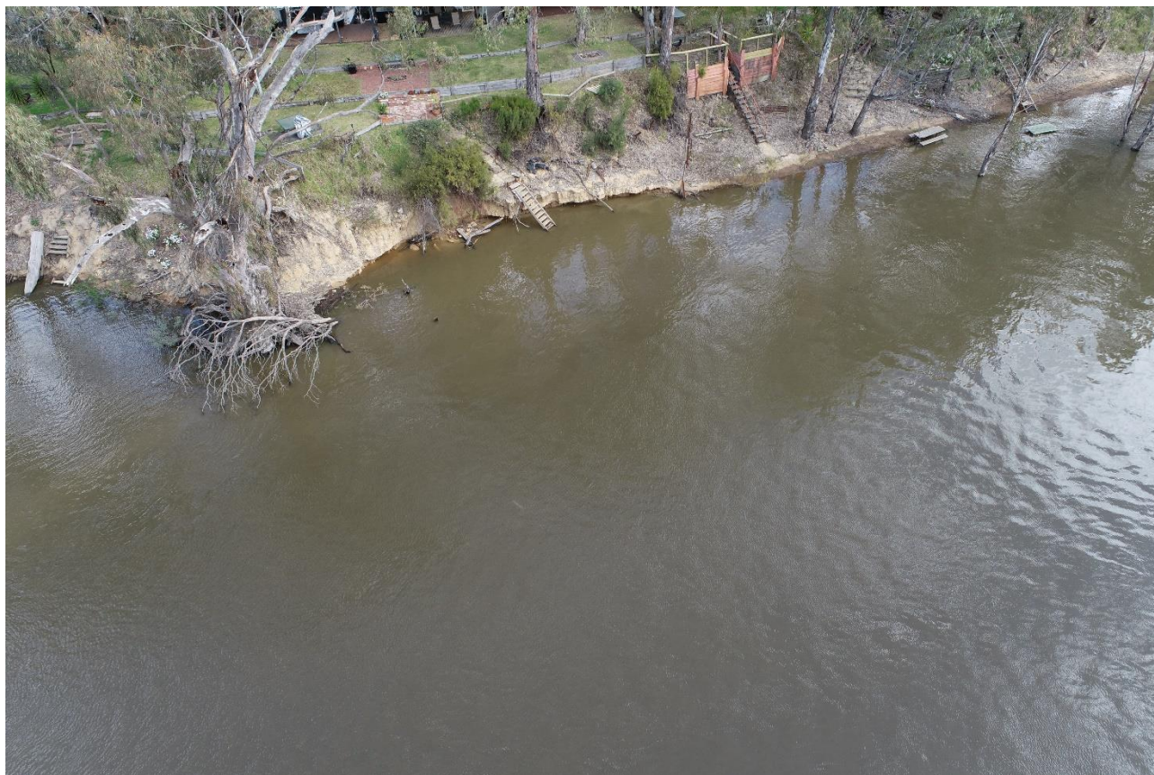
Figure 2: Site 1 – riverbank erosion (eroded toe, causing bank failure)
